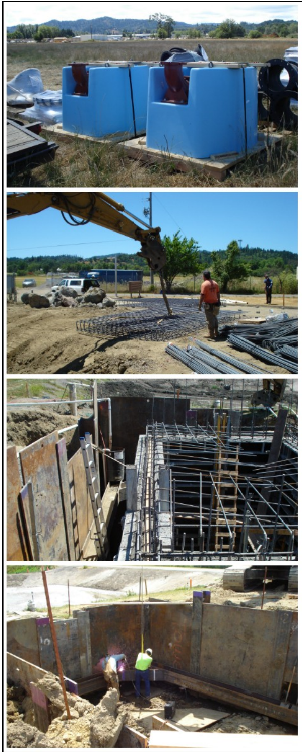
Various construction activities at the Willits WWTP, including: wet well pump bases before placement, rebar fabrication for the wet well and foundation of the head works building, and installation of wet well pumps.
