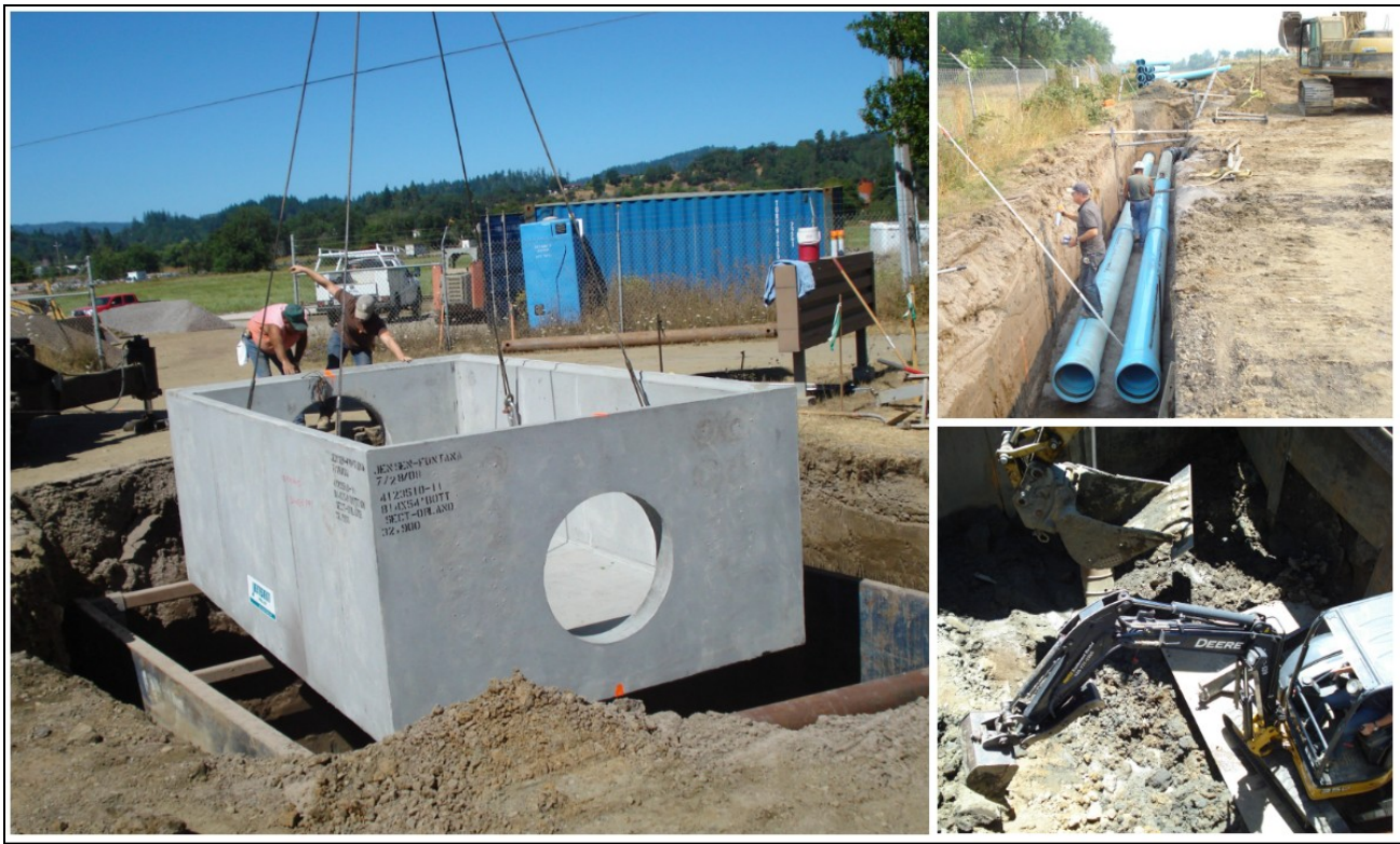
Various construction activities at the Willits WWTP, including: effluent distribution weir placement, 16-inch influent and effluent lines to the aeration basins, and excavation of the (+/-) 20-foot-deep wet well for the project headworks.
