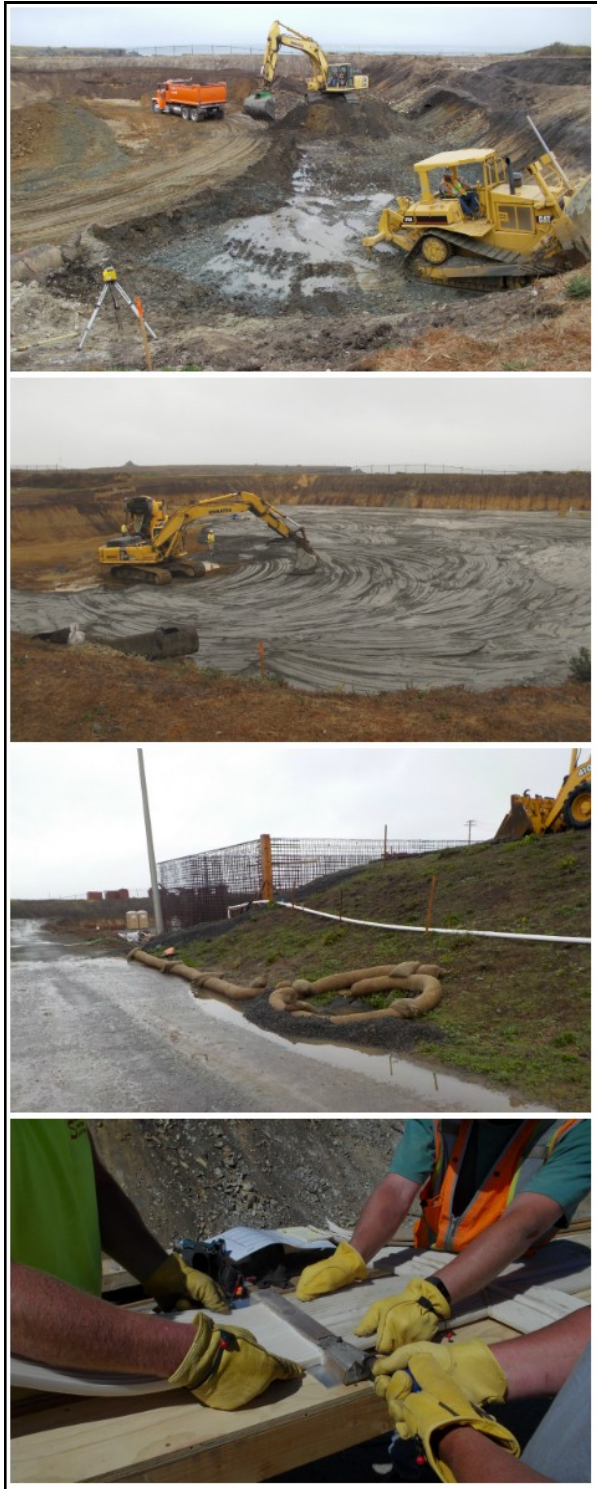
To date, SHN is proud to report that the Fort Bragg WWTP project has proceeded ahead of schedule and under budget.
