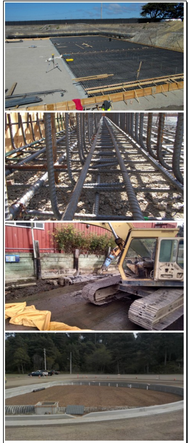
Project photography from two recent SHN projects within Fort Bragg (the new WWTP construction and the harbor boat-launch facility).
