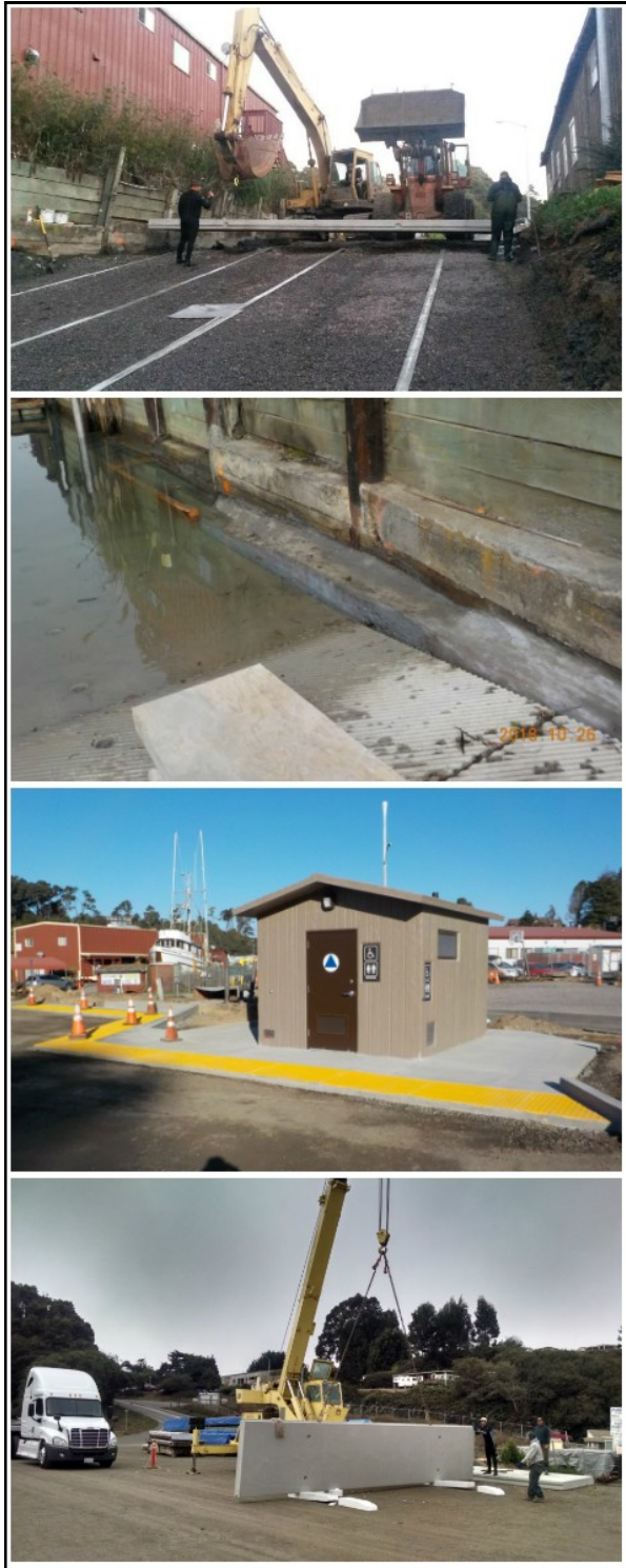
The new ramp extends farther into the river and should make for an easier time getting vessels into and out of the water. Also the new parking lot will feature a circular 4,500-square-foot “bioretention area,” essentially a large drain with soil and gravel filters to treat surface water running over the asphalt and into the river.
