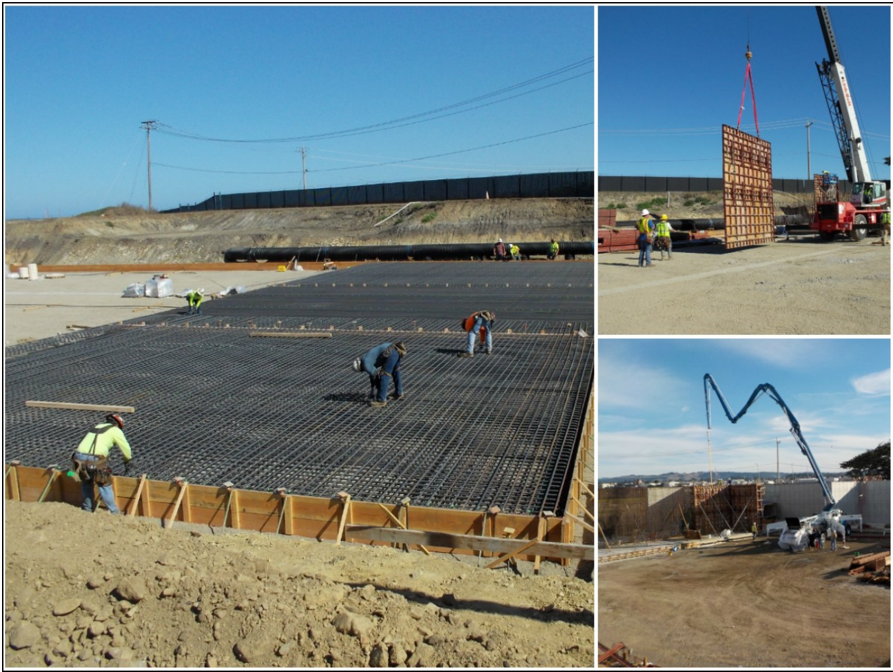
The Fort Bragg WWTP project has included various elements of construction management and inspection services, including a strict adherence to management of American Iron and Steel certifications and tracking.
