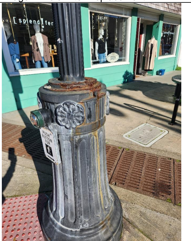
Image 4: Current Condition of other poles at Intersection
