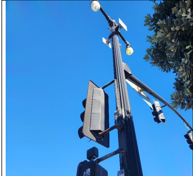
Image 5: Current Condition of other poles at Intersection
