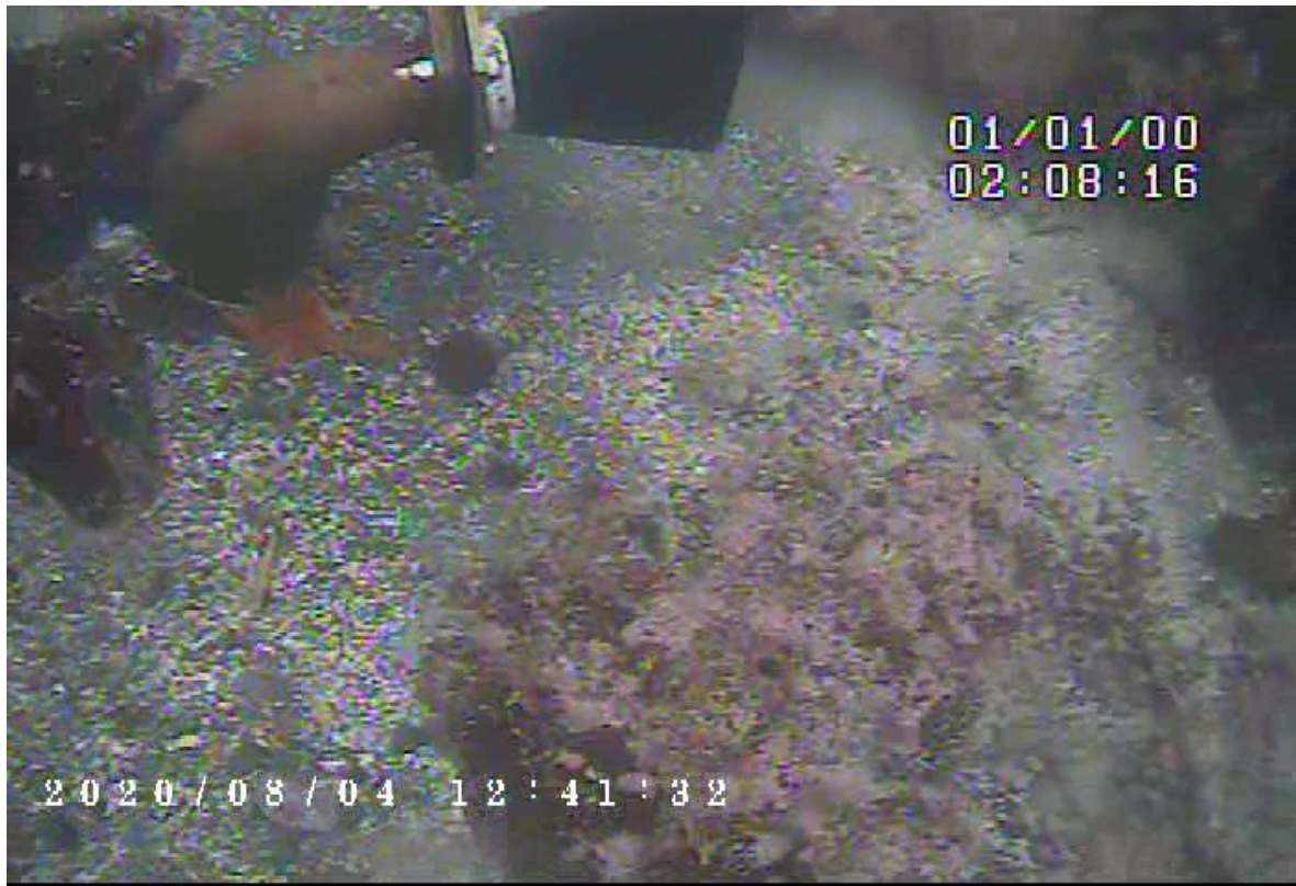
Photo 5 – Diffuser 11 showing strong flow
