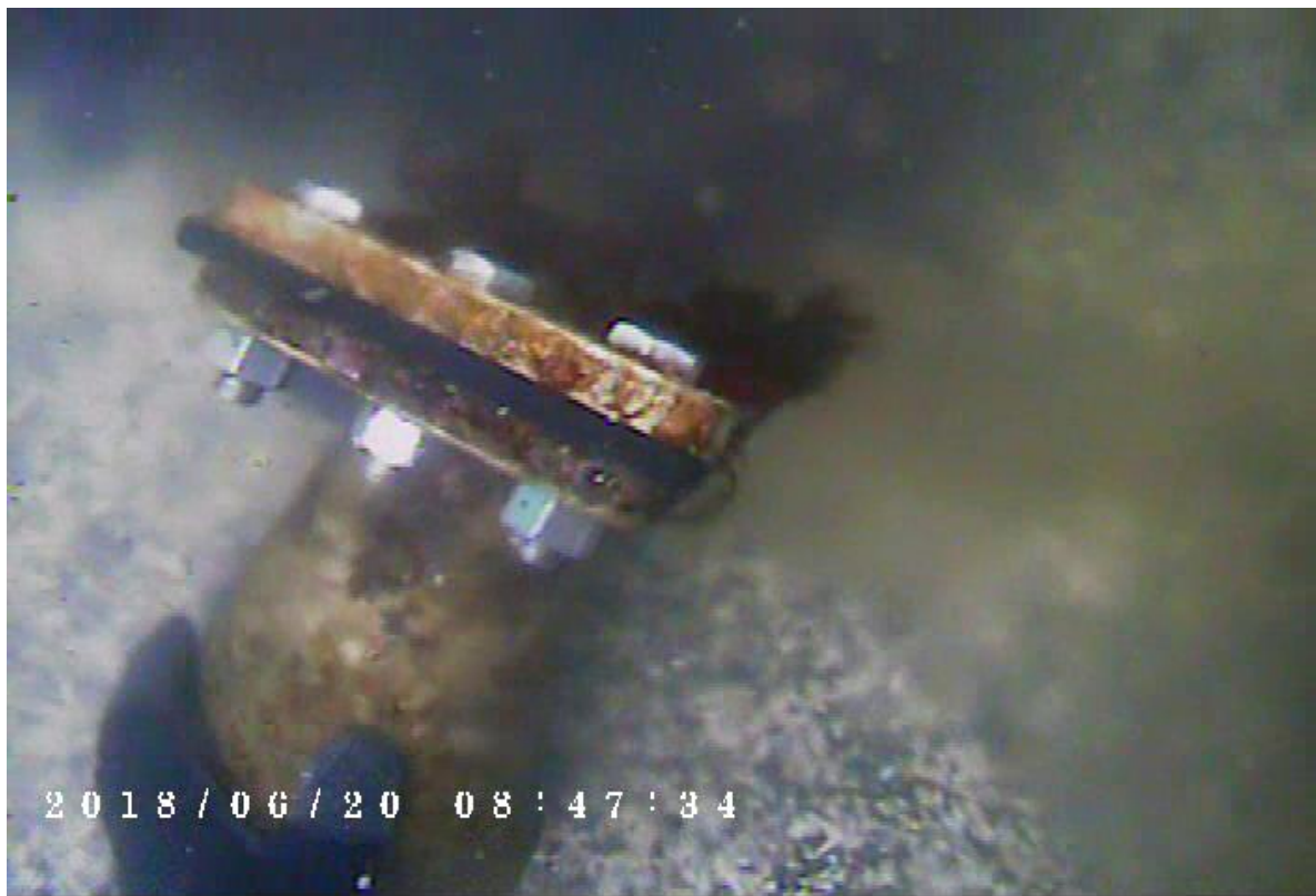
Photo 10 – Diffuser 10 showing strong flow
