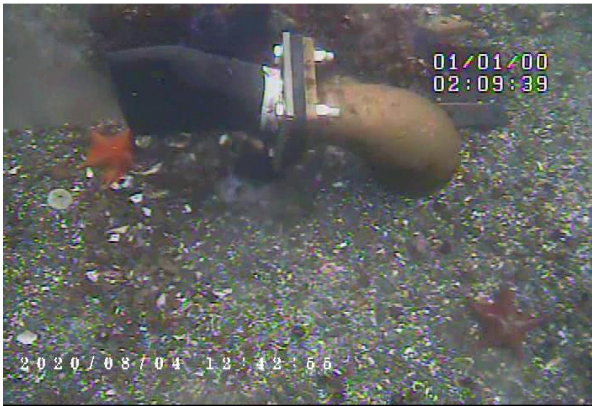
Photo 10 – Diffuser 6 showing strong flow
