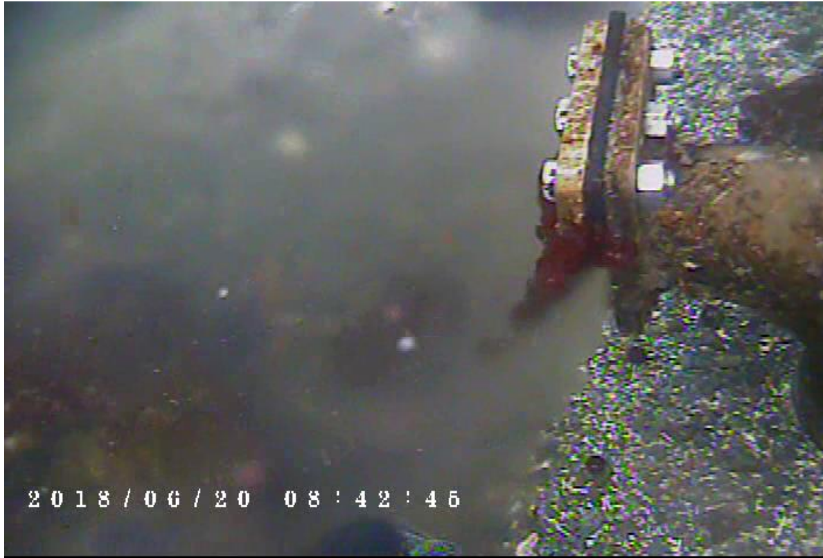
Photo 3 – Diffuser 3 showing strong flow
