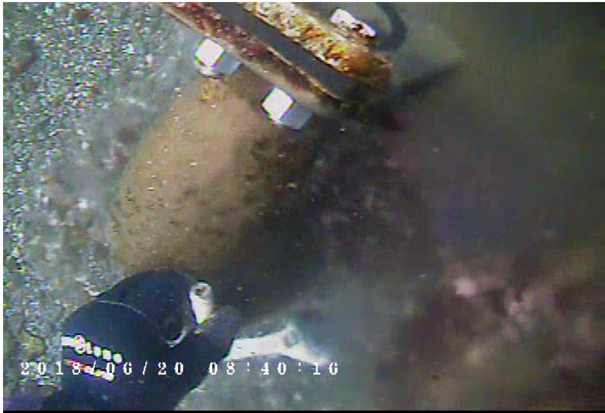
Photo 1 – Diffuser 1 showing strong flow
