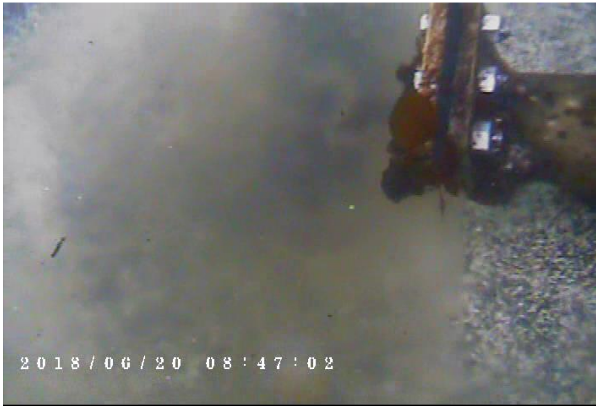
Photo 9 – Diffuser 9 showing strong flow
