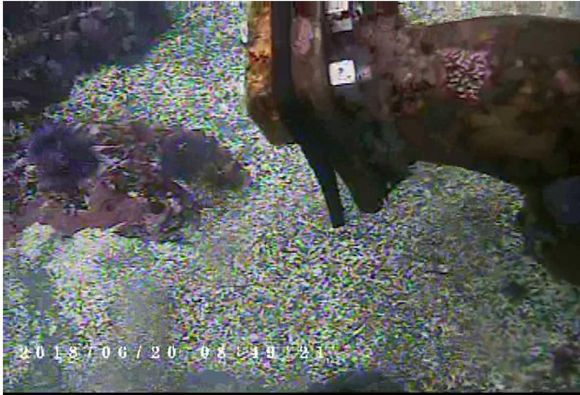
Photo 13 – Diffuser 13 showing light flow
