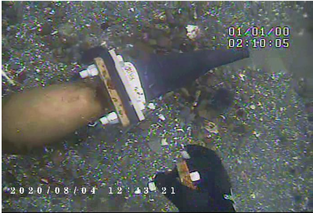
Photo 11 – Diffuser 5 showing strong flow
