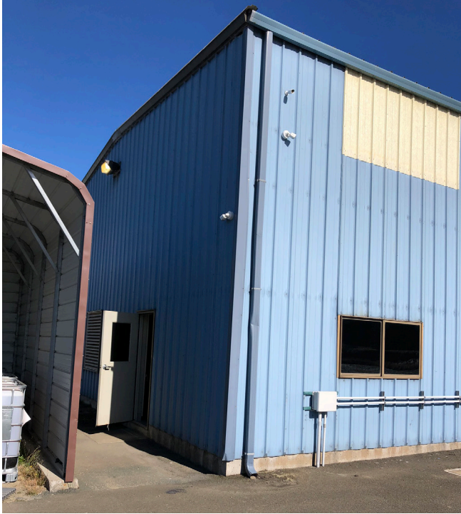
The corner of the control building is settling, so HDR's geotechnical engineer will perform a qualitative assessment of the settlement issues to figure out how to mitigate.
