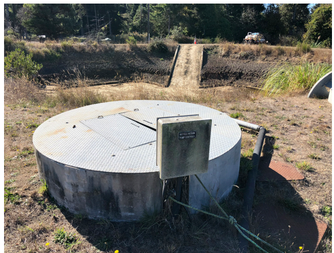
Pipe penetrations are leaking back to the raw water ponds.
