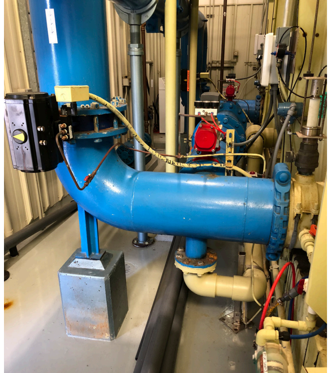
The filter-to-waste line is too small and needs to be increased.
