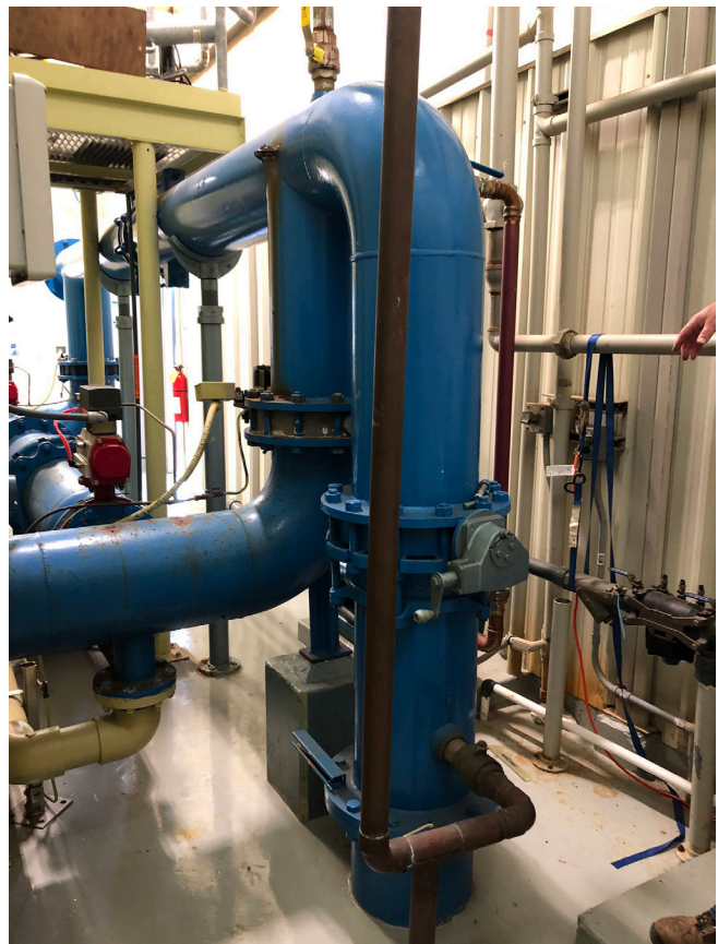
A flow meter needs to be installed.
