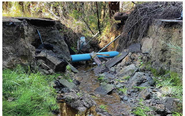
Fort Bragg - Brush Creek Atmospheric river culvert failure
