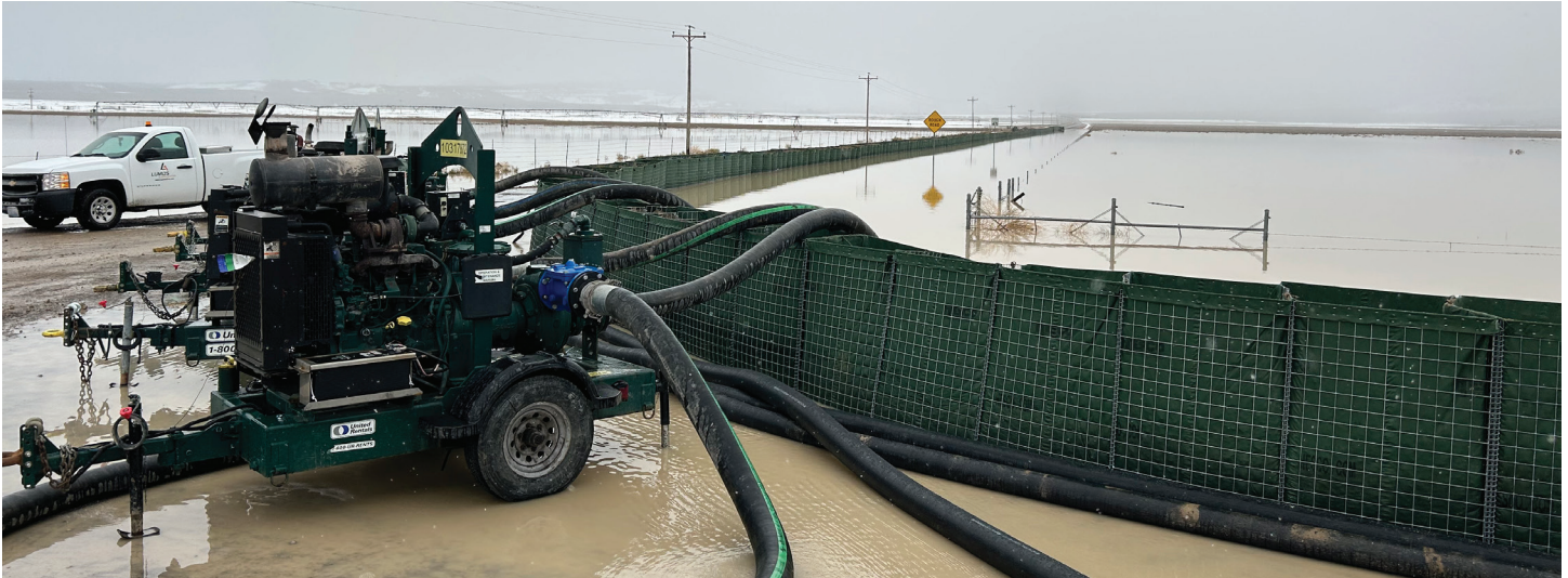
Lumos' flood mitigation solutions during Eureka County's 2023 emergency event
