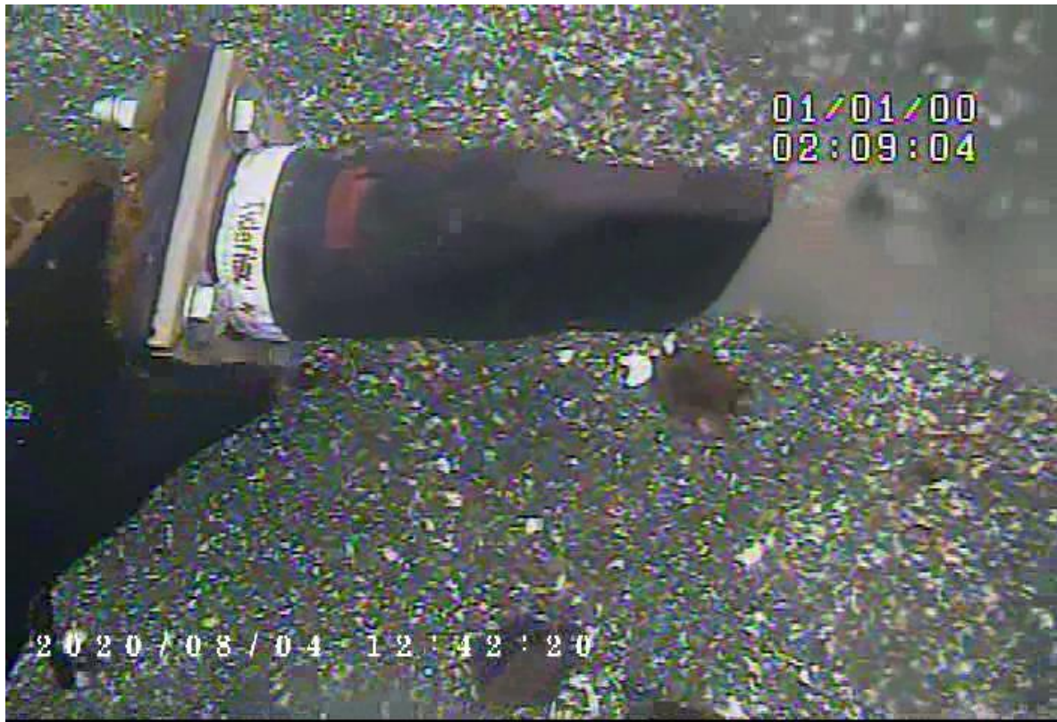
Photo 7 – Diffuser 9 showing strong flow
