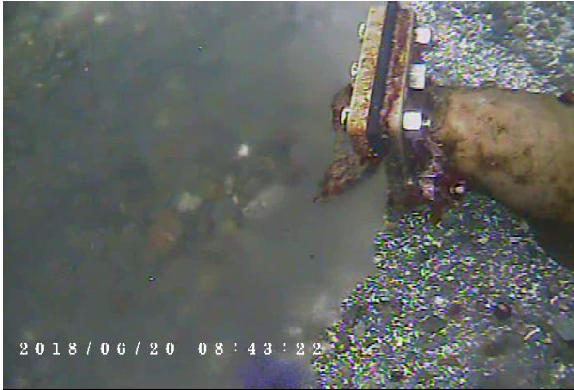
Photo 5 – Diffuser 5 showing strong flow
