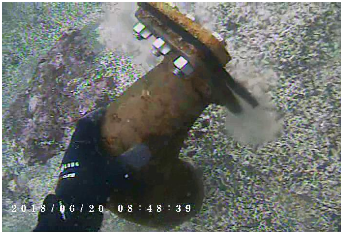
Photo 12 – Diffuser 12 showing light flow
