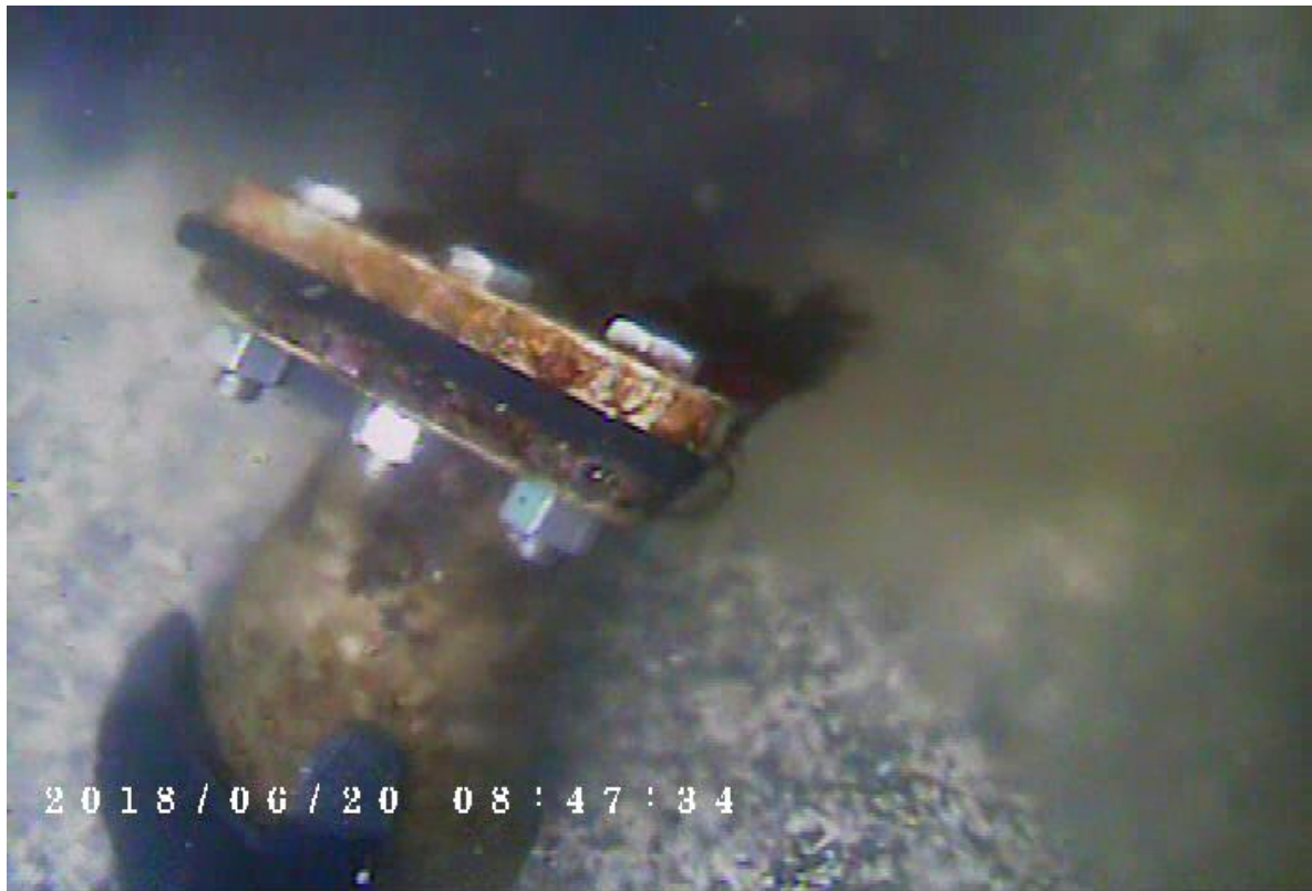
Photo 10 – Diffuser 10 showing strong flow
