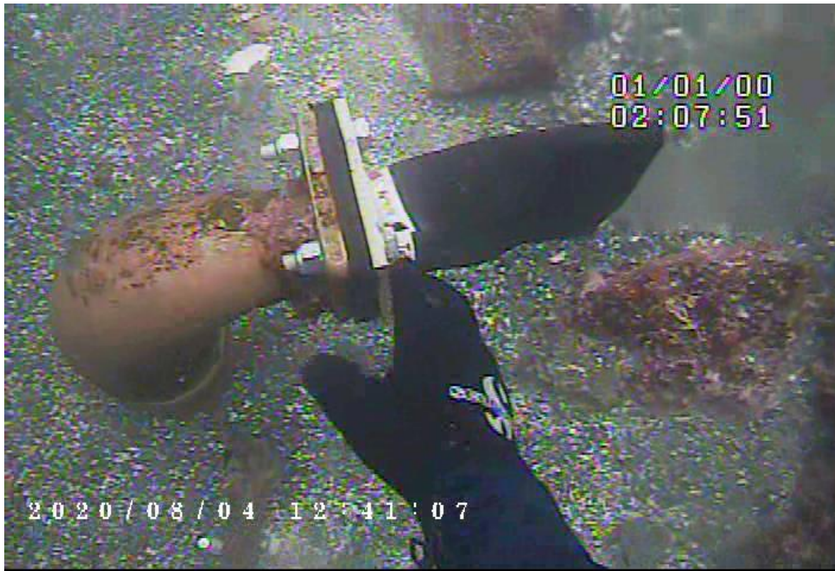
Photo 3 – Diffuser 13 showing strong flow
