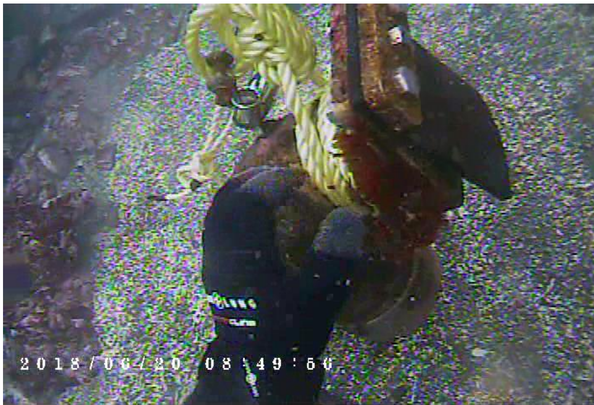
Photo 14 – Diffuser 14 showing no flow
