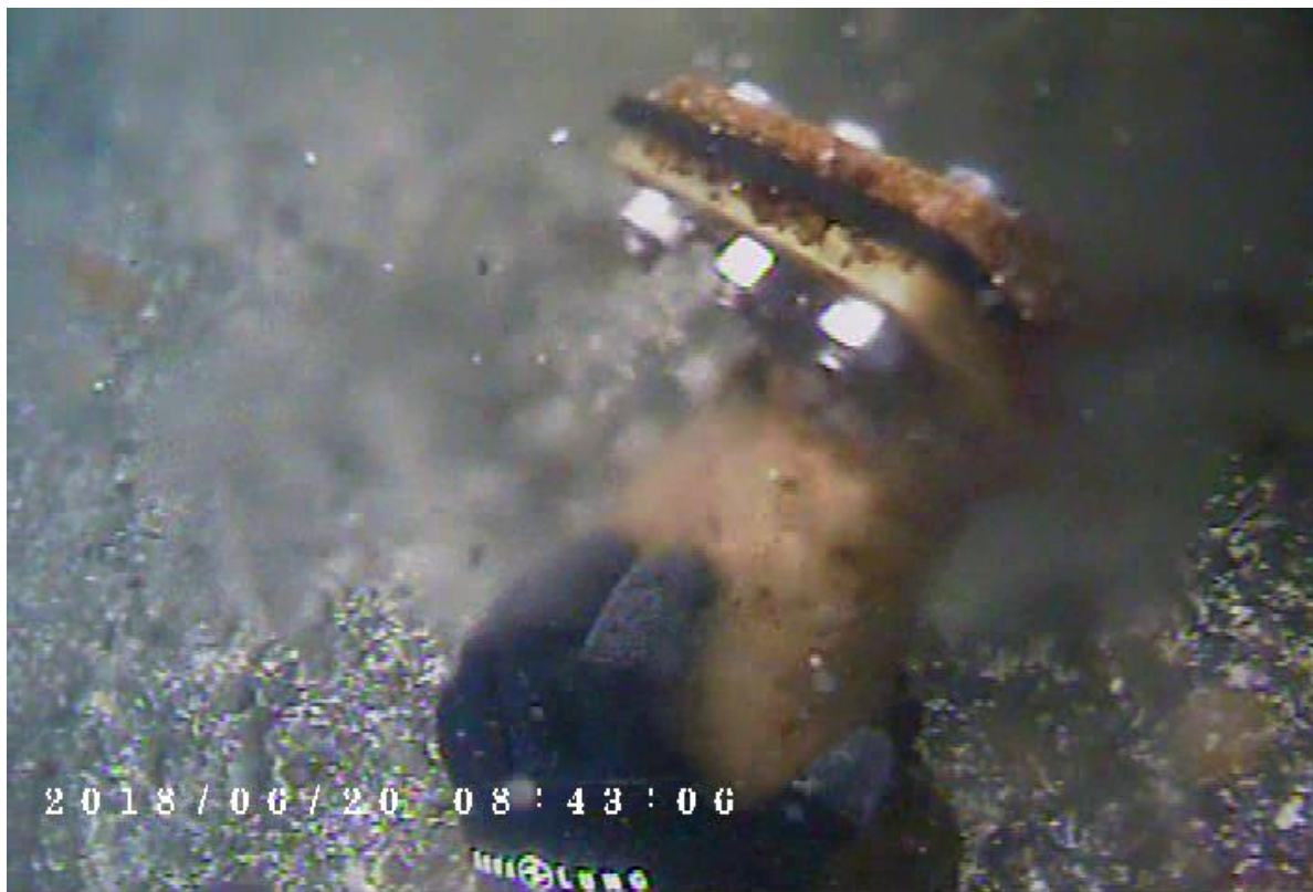
Photo 4 – Diffuser 4 showing strong flow
