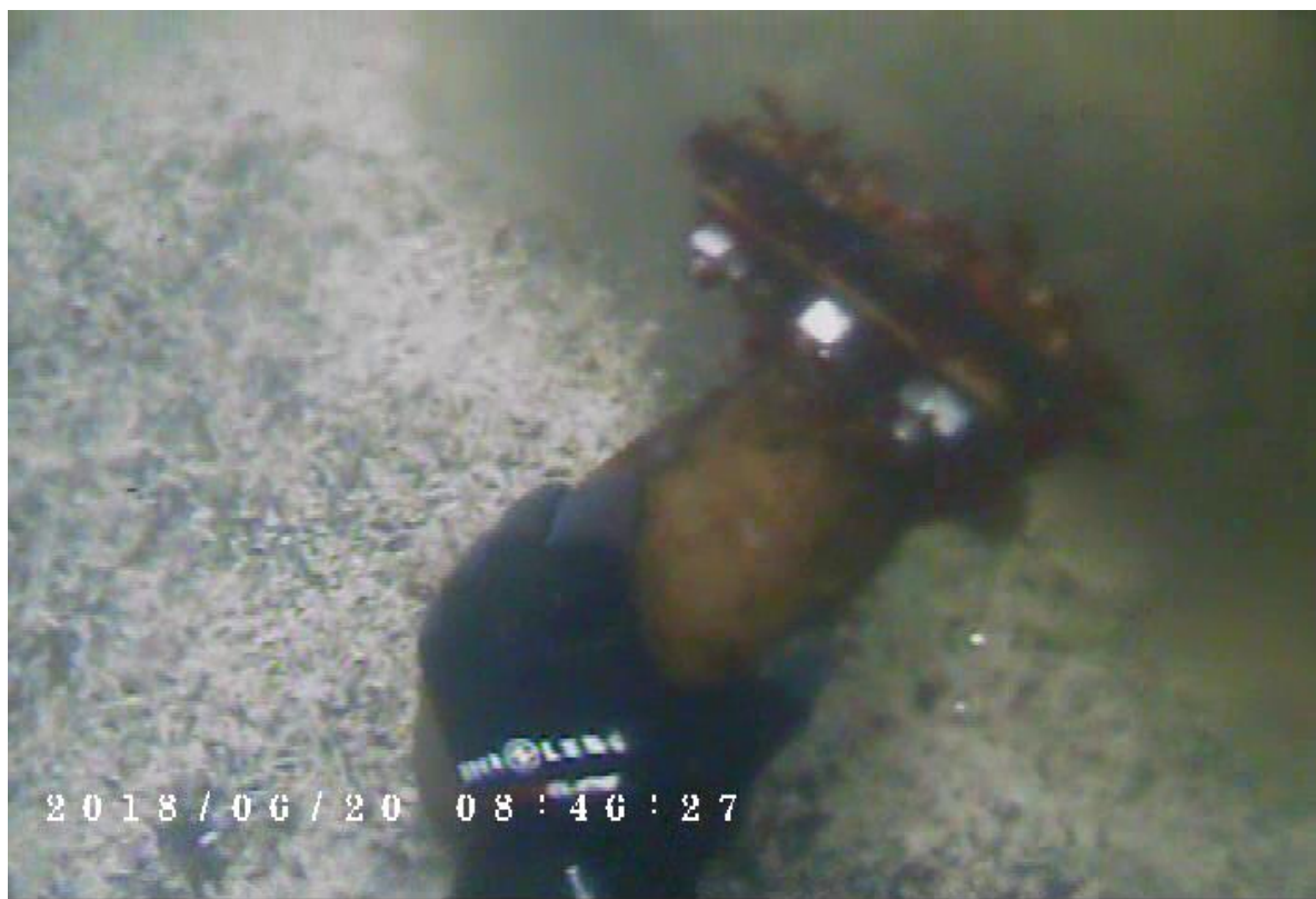
Photo 8 – Diffuser 8 showing strong flow
