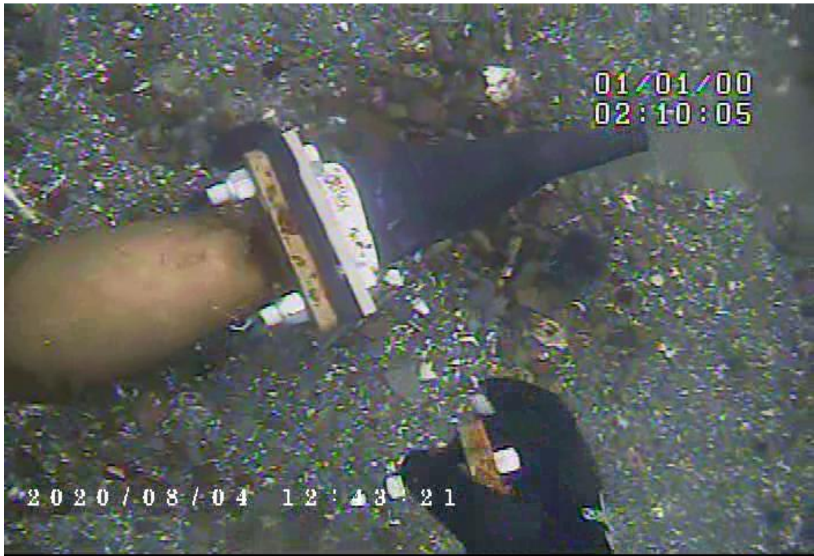
Photo 11 – Diffuser 5 showing strong flow
