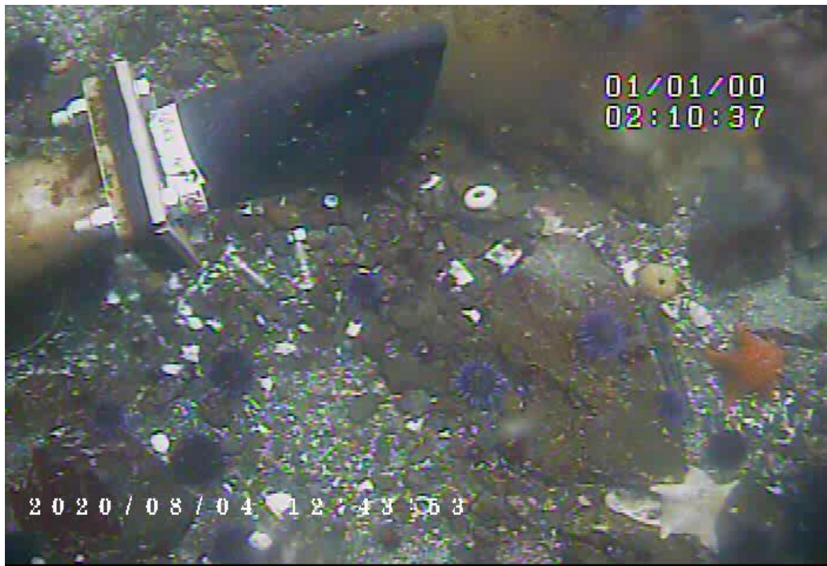
Photo 13 – Diffuser 3 showing strong flow
