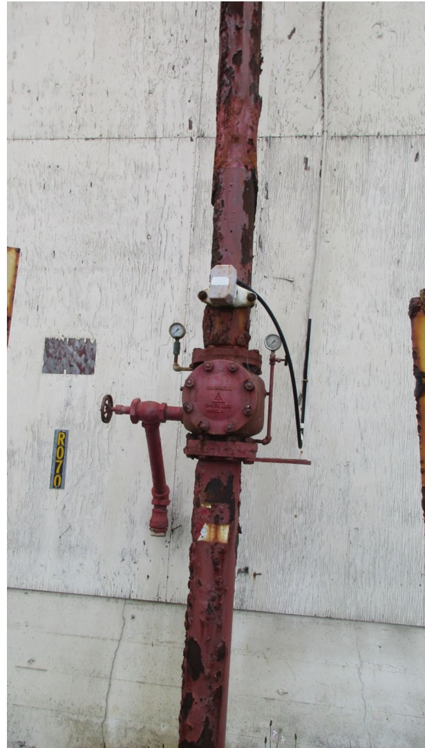
Deteriorated sprinkler main
