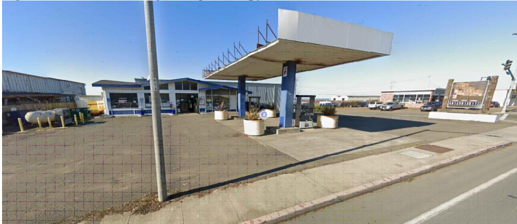
Figure 2: Photo illustrating damaged canopy
