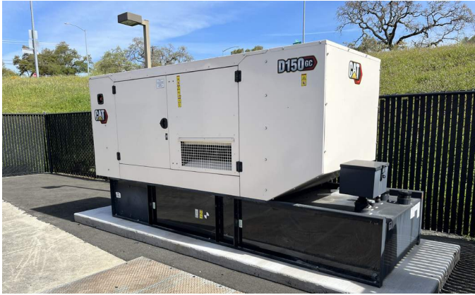
City of Santa Rosa New Backup Generator
