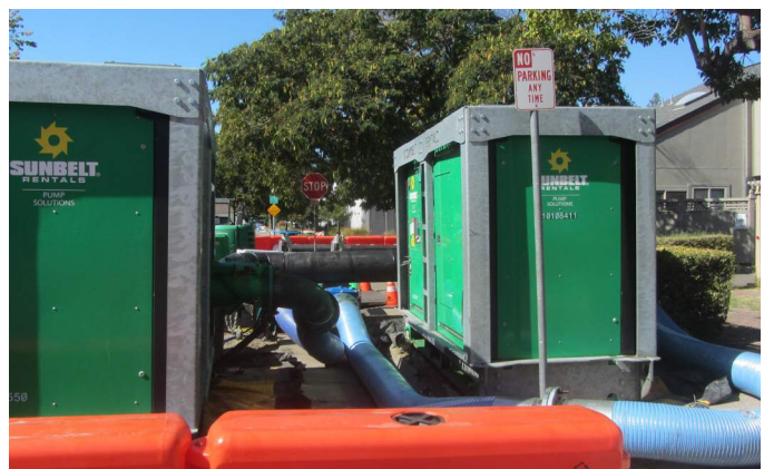
Temporary Bypass Pumping for the City of Santa Rosa Crosstown Trunk Sewer Replacement
