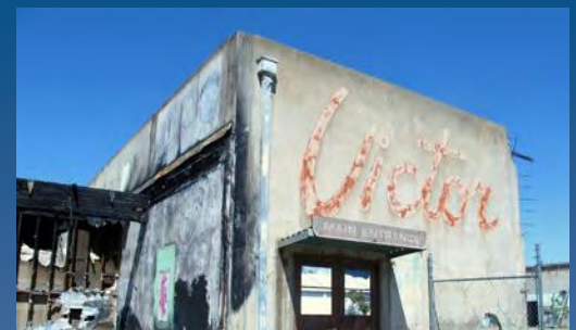
Chico is working to redevelop this key brownfield site as part of a larger effort to support green companies in "The Wedge" business area.
