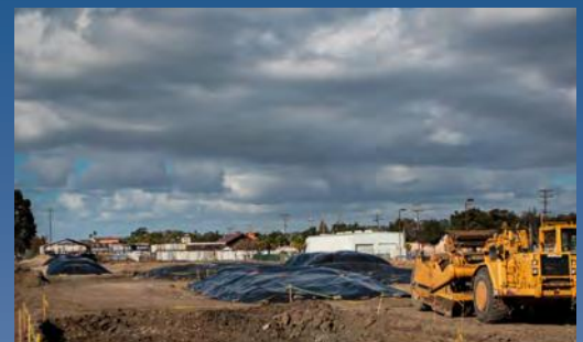
Contaminated soil is removed at the 4.5 acre site that is now the Rumrill Sports Complex.
