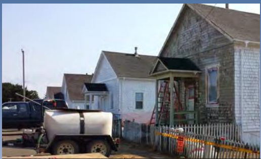
Lead-based paint that peeled off old homes in the historic mill town of Samoa created a health hazard by contaminating soil in the surrounding area.
