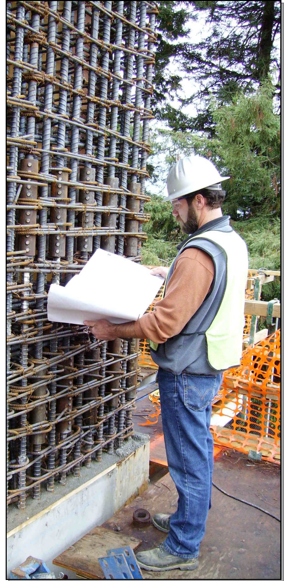
SHN inspector verifying rebar placement and dimensions to assure consistence with project plans.
