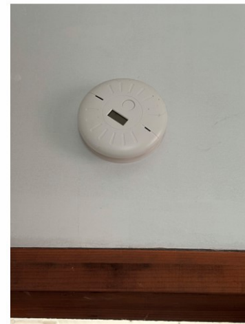
Typical Fire Alarm throughout 2 bldgs
