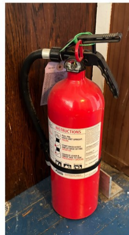
Typ. Fire Extinguisher throughout 2 bldgs
