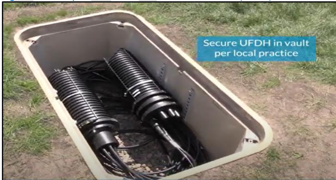
Figure 5 – Example of Universal Fiber Distribution Hub (UFDH) in vault
