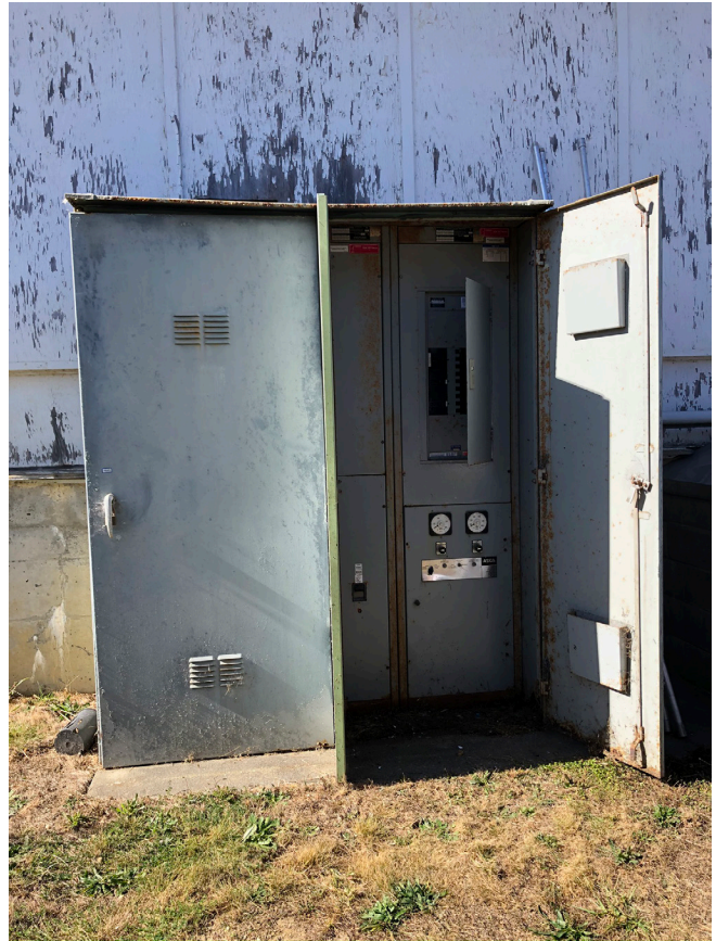
Electrical panel (main switchgear for Plant where Pacific Gas & Electric [PG&E] Feed Comes in) needs to be replaced.
