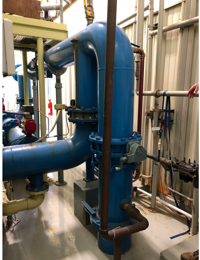
A flow meter needs to be installed.
