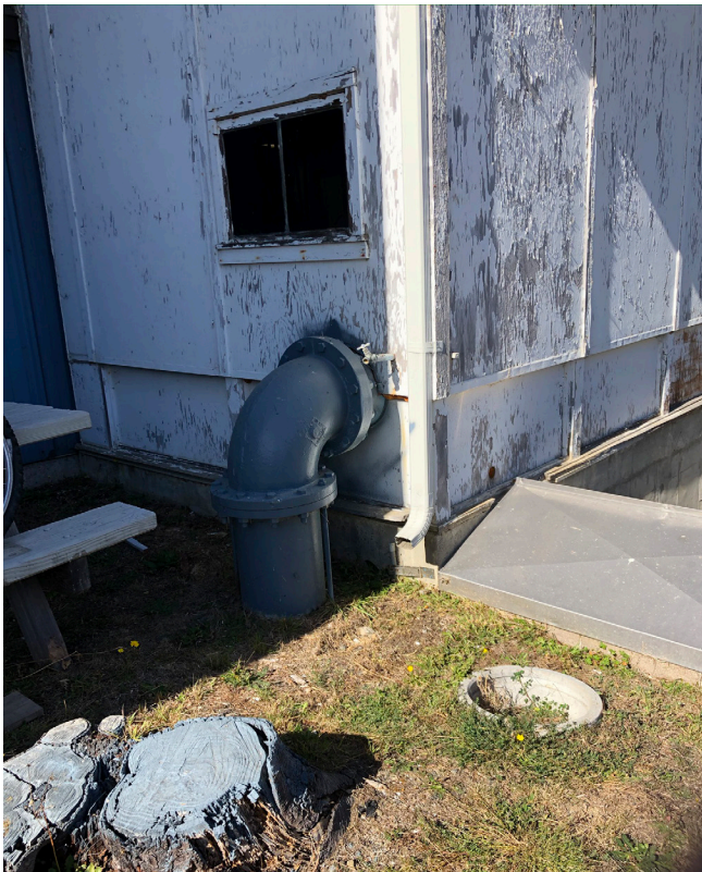
Pipe is settling and needs to be excavated and stabilized.
