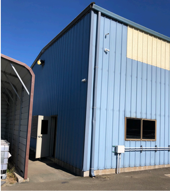
The corner of the control building is settling, so HDR's geotechnical engineer will perform a qualitative assessment of the settlement issues to figure out how to mitigate.
