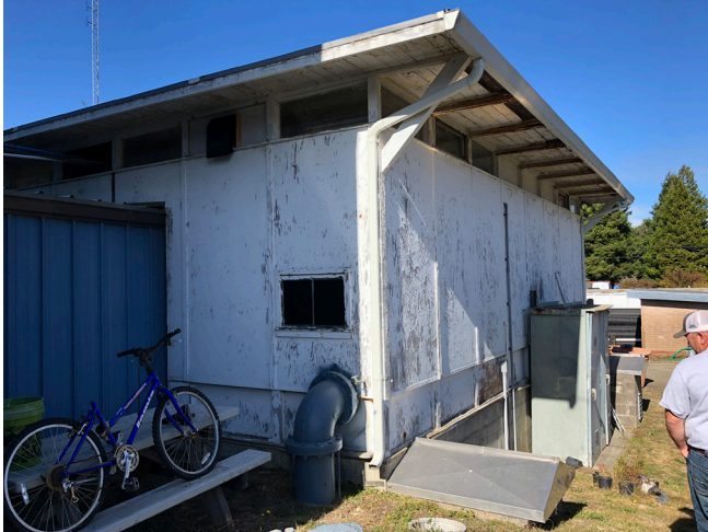
The entire wood building needs to be demolished and replaced with a pre-engineered metal building.
