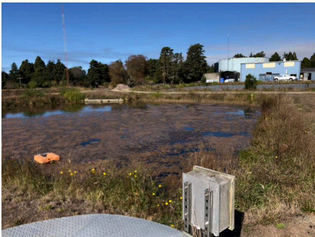
Raw water ponds are leaking and need HDPE liner.
