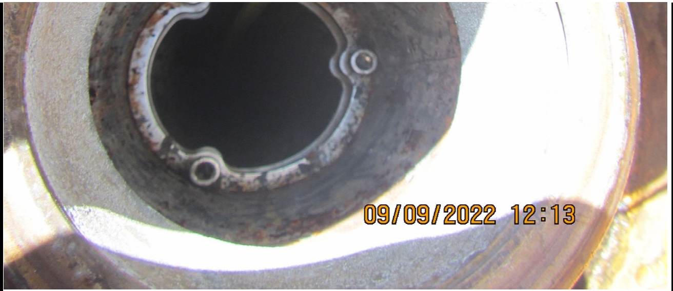
Photo No. IMG_0025-Tape measurement of product level inside tank two, eastern tank
