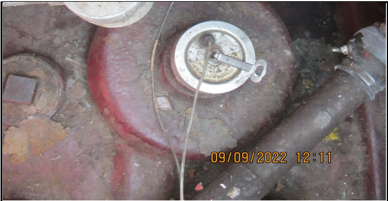
Photo No. IMG_0024-Close-up of annular space sensor riser for tank two, eastern tank
