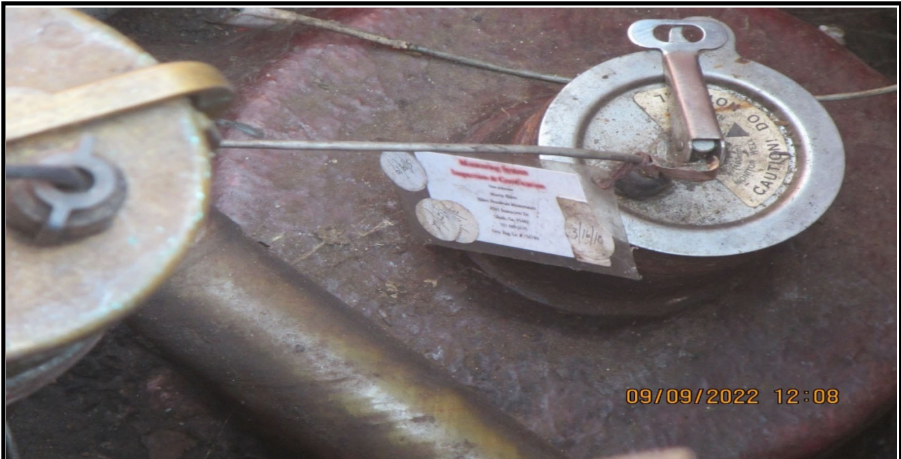
Photo No. IMG_0014-Close-up of annular space sensor riser for tank one, western tank
