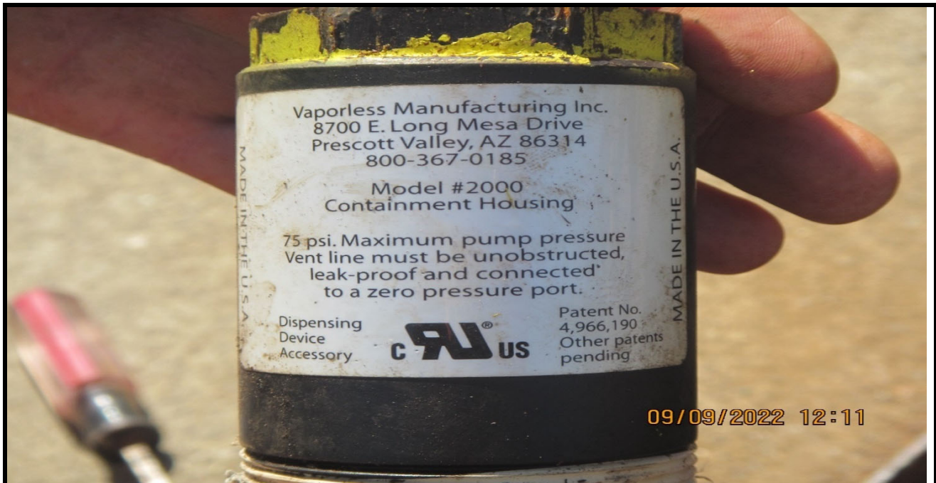
Photo No. IMG_0022-Close-up of LLD inside tank two, eastern turbine sump
