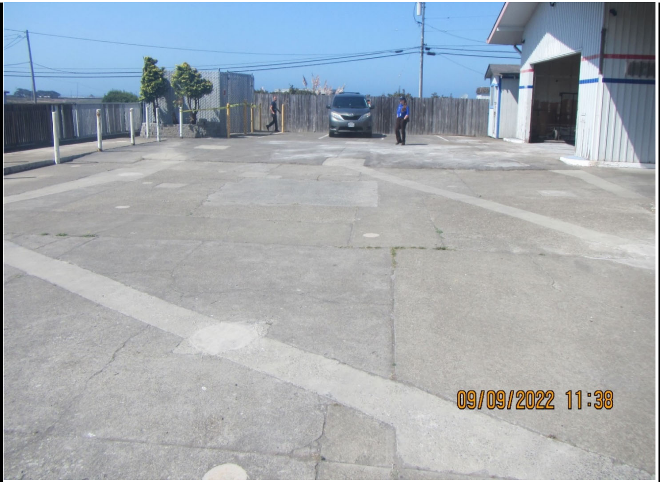
Photo No. IMG_0005-Overview of pavement patches from former site remediation and investigation events.
