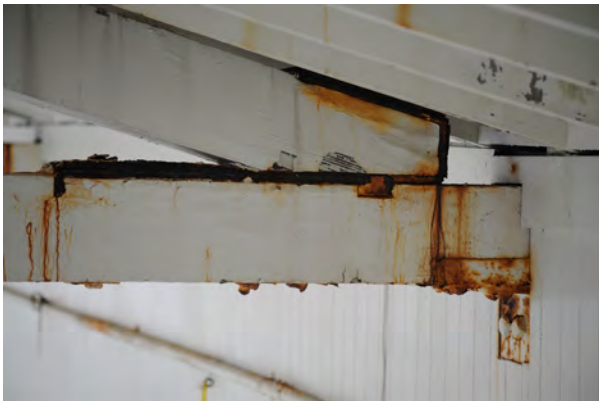
HEAVILY CORRODED POOL TRUSS HEEL CONNECTION
