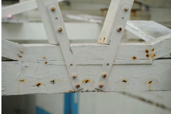
POOL TRUSS SHOWING FORMER REPAIR WORK
