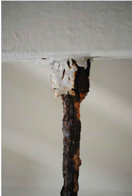
HEAVILY CORRODED STEEL ROD SUPPORT HANGERS AT CATWALK
