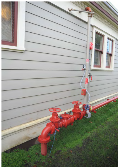
FIRE SPRINKLER RISER SERVING CITY HALL EAST
