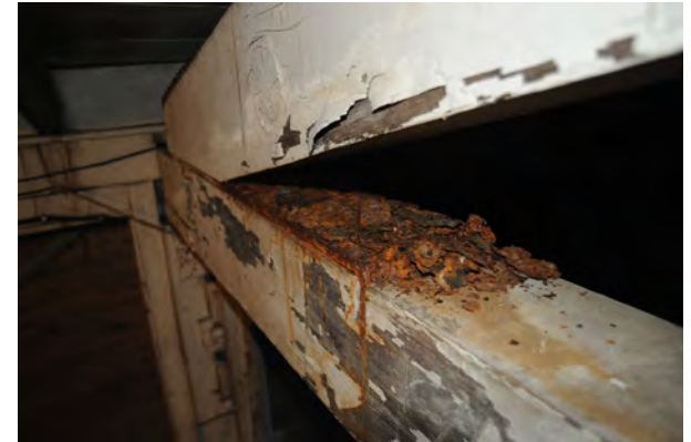
HEAVILY CORRODED POOL TRUSS HEEL CONNECTION IN SOUTH WING LOW BAY SPACE
