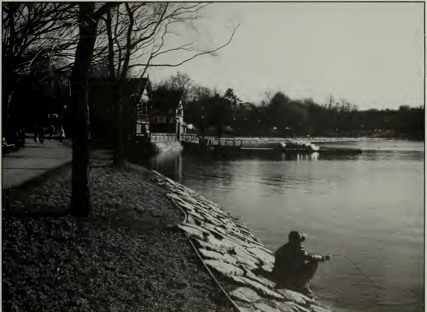
Jamaica Pond has an ongoing erosion problem, exacerbated by wave action. To stabilize the shoreline, this stone rip-rap was modeled after the original detail implemented by the Olmsted firm. (Pressley Associates and Boston Parks & Recreation)
