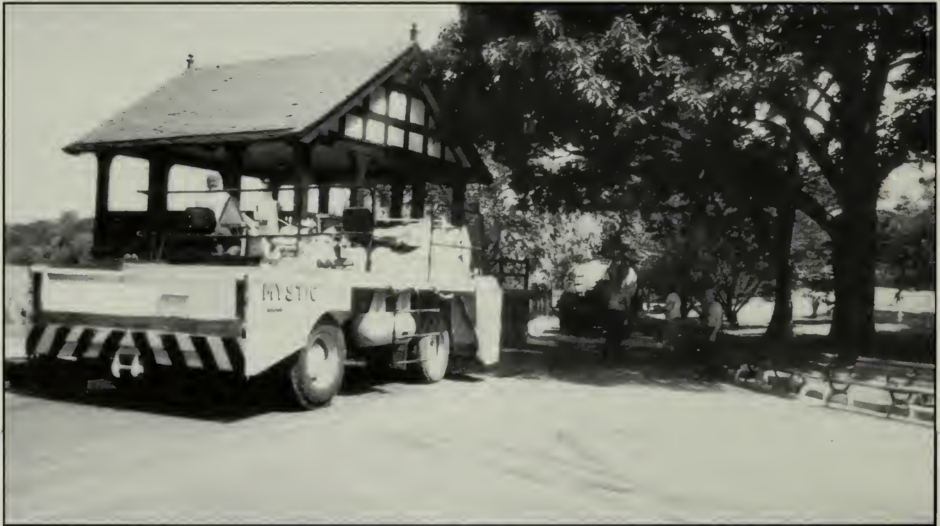
As part of a preservation project, the walks around Boston's Jamaica Pond Park were repaired and resurfaced. A loose, crushed stone surface material (an embedded aggregate) was rolled into the asphalt surface, thus allowing for upgraded uses such as jogging, biking and snow removal, while retaining the historic character. (FLONHS and author, 1990)
