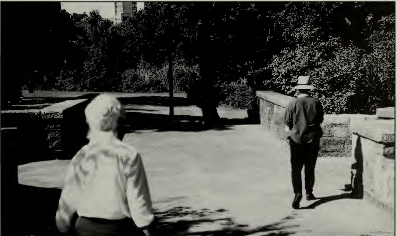
Many of the stones from the Island Bridge along Boston's Riverway had fallen into the Muddy River below. As part of the preservation work, these stones were retrieved from the water and reused, in addition to several new stones that were cut to order to replace in-kind those that were lost. (author, 1988, 1994)
