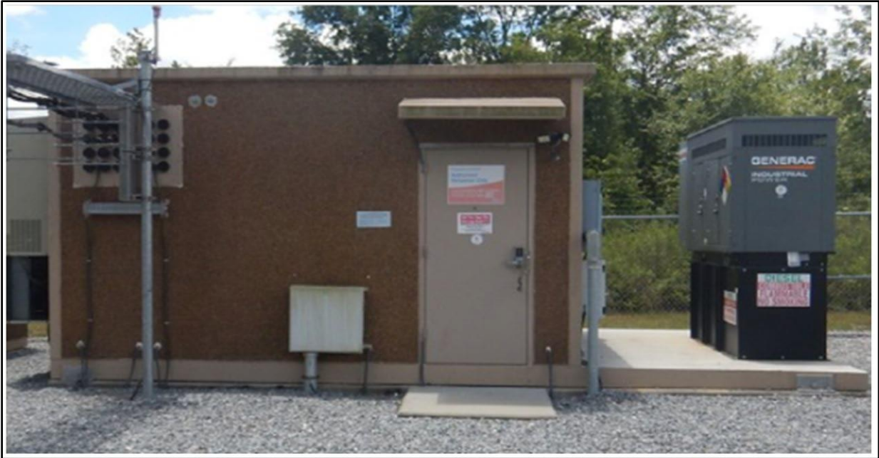
Figure 8. Network Hub with Diesel Backup Generator
