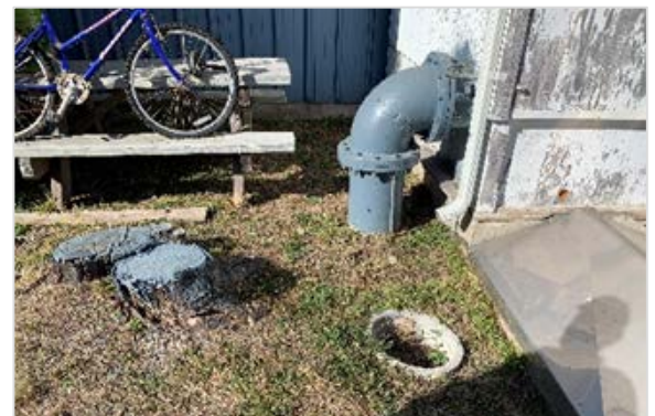
Settled pipe after tree removal
