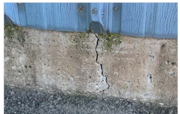
Crack in the filter treatment building slab
