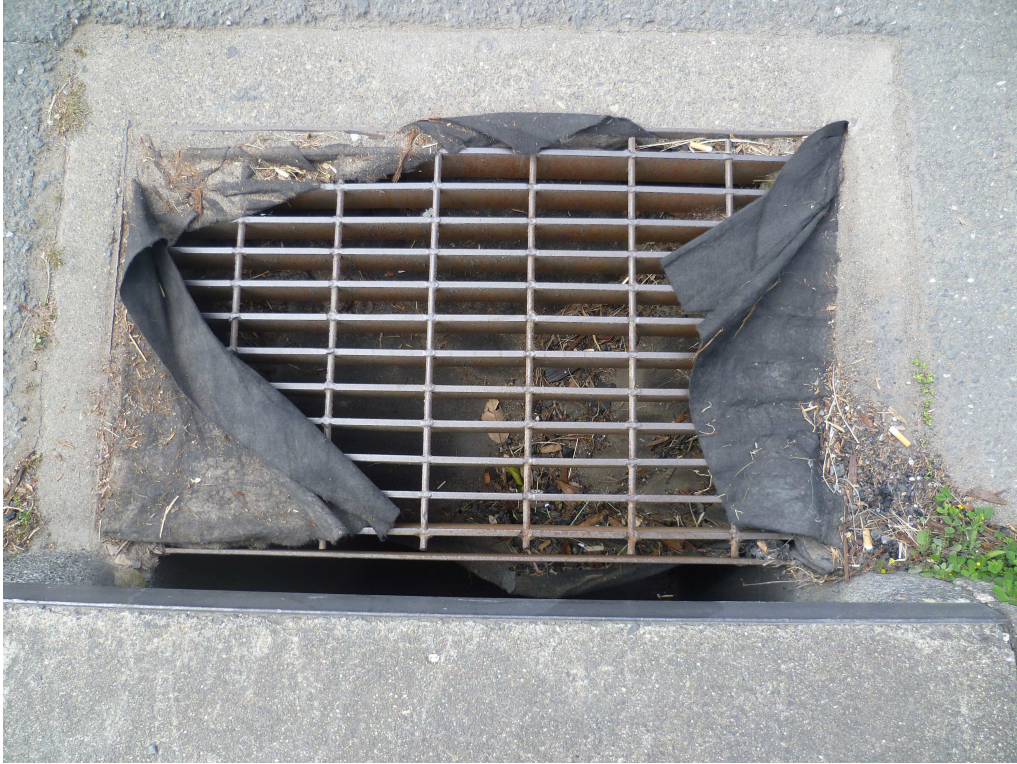
CalTrans sheathing from roadwork never removed
