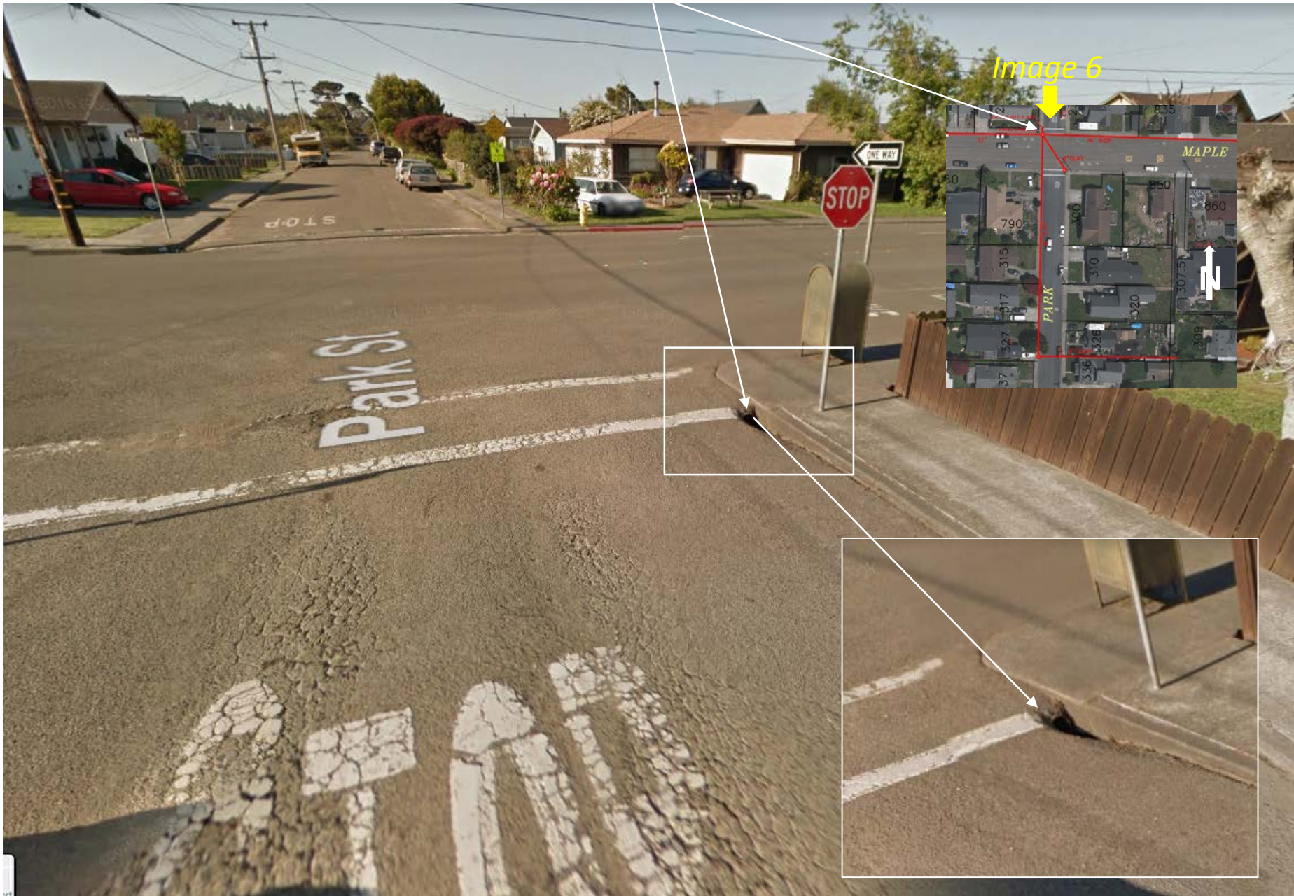
Image 6 - Inlet (pipe opening only) at NW corner Park and Maple – view looking south
