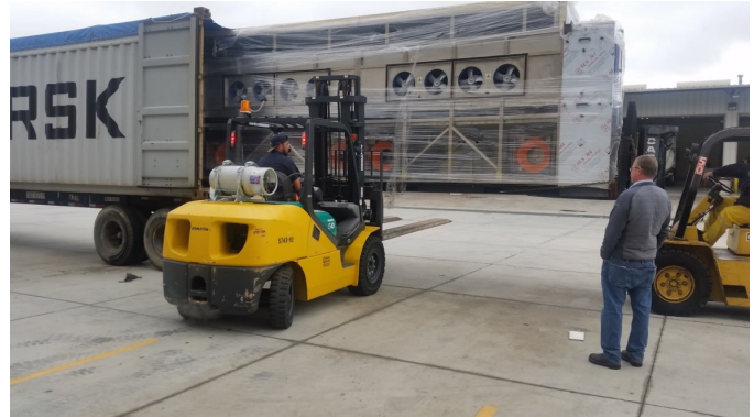
Second Forklift placed underneath Belt Conveyor
